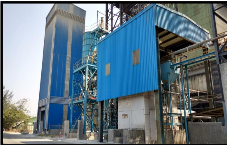
Ash Grinding Unit & 300 MT Silo
