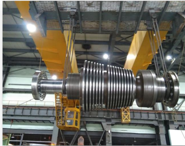
Refurbished IP turbine
