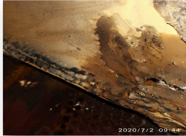
HPH-5 LHS Outer side base plate eroded.
